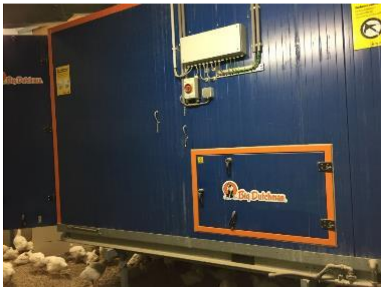
Figure 11: Picture by Author. Heat Exchanger in outdoor access area for chickens.
