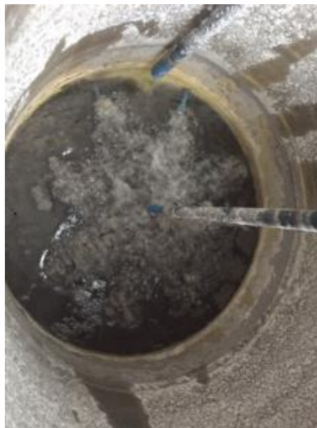
Figure 39: Perforated pipes pumped with air for mixing (Author)
