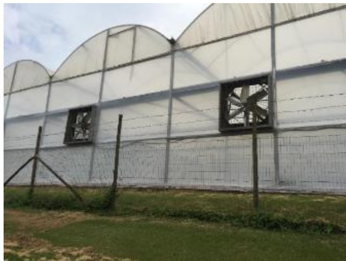
Figure 21: Evaporative cooling system, Holambra, Brazil (Author)
