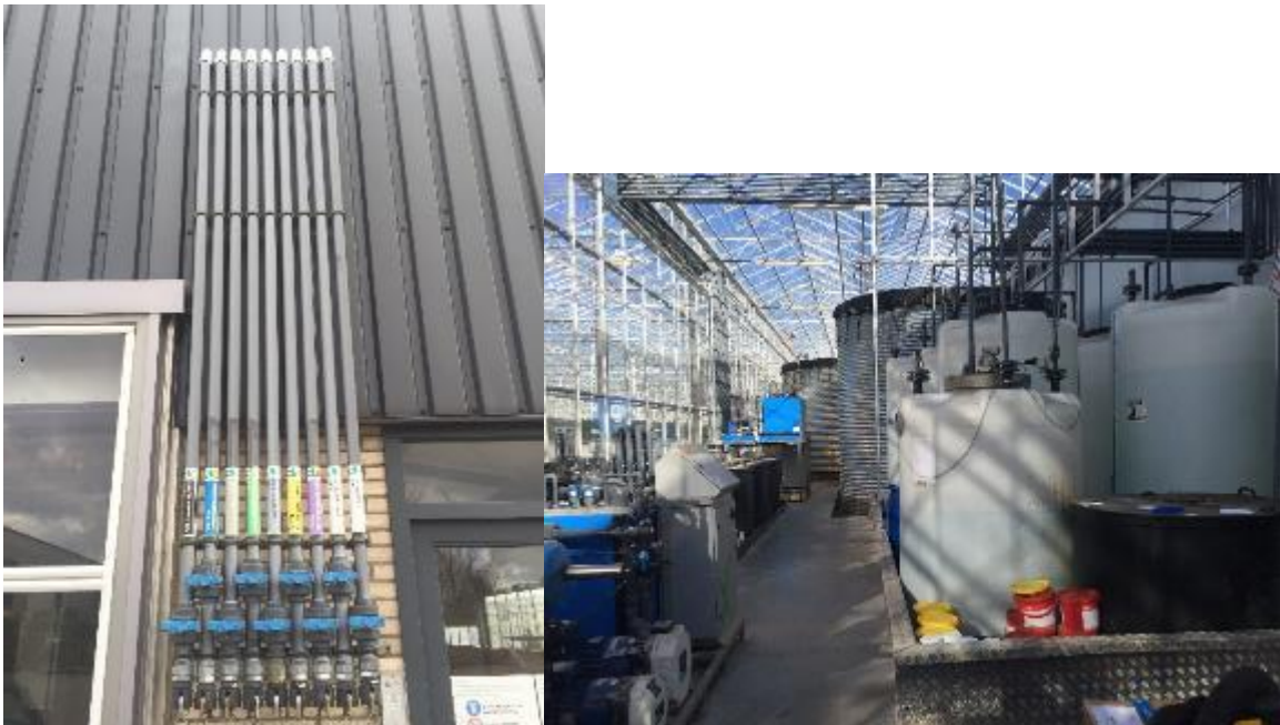
Figure 40: Fertiliser tanks in Netherlands (Author)
