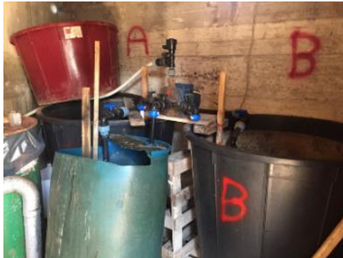
Figure 36: One dose pump to run both A tank and B tank fertilisers (slug dosing)
