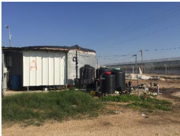
Figure 41: In Israel, black tanks are outside and depending on set mixes whether vegetative or regenerative, orders get delivered to site.
