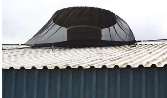
Figure 13: Fly netting is installed on fans during summer months
