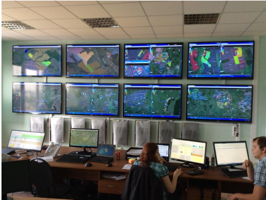
Figure 8.1: Central control room at Black Earth Farms.
