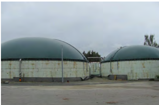
Figure 11: The bio-digester installed on the Ottilien Monastery.
