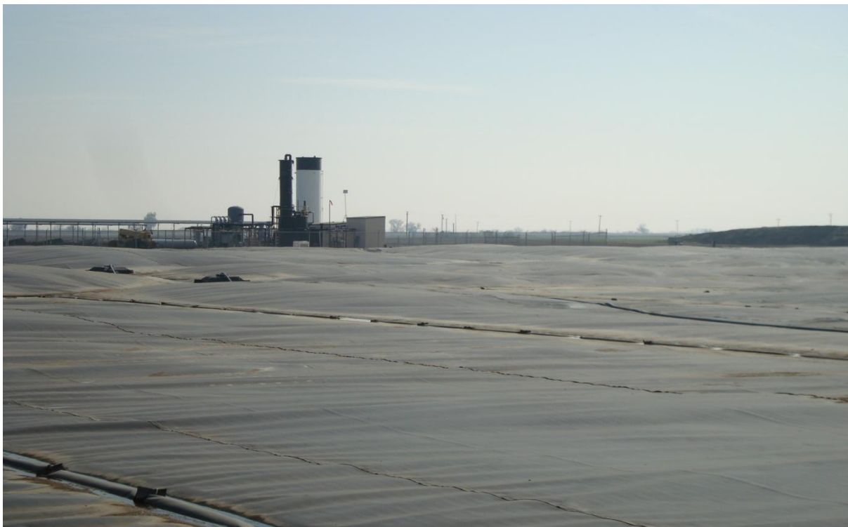
Vintage Dairy, Fresno California. BioEnergy's first methane capture unit. The covered slurry pit has the optimum 42 days capacity. The scrubber can be seen in the background.
