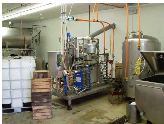
18 Jim Koan's Cider plant, Flint Michigan USA
