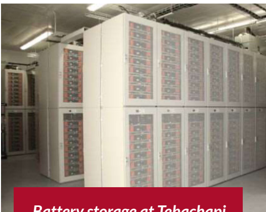
Battery storage at Tehachapi
