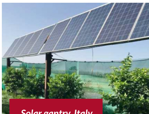
Solar gantry, Italy
