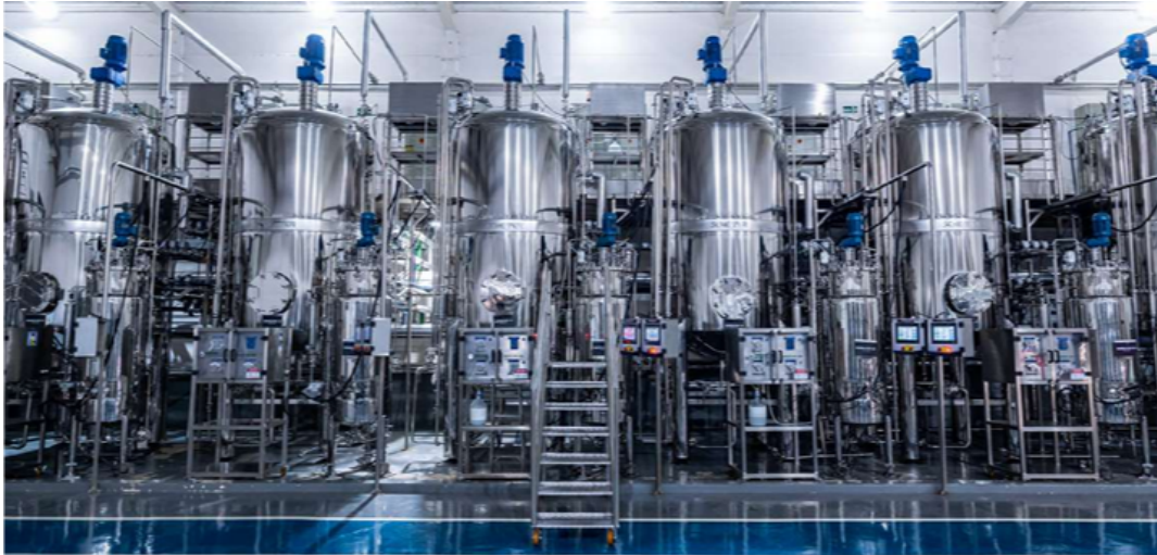
Figure 18 The facility used to brew their biological inputs (Source: Author)
