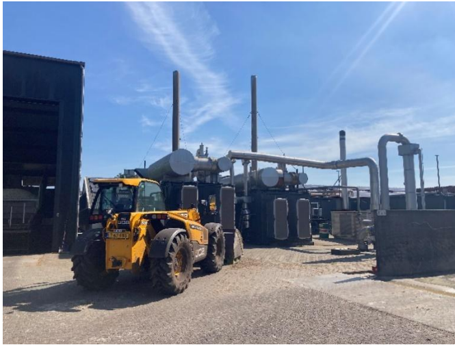
Figure 9. Two large generators running on biogas to produce electricity. Source Author's own
