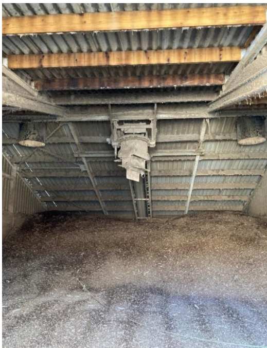
Figure 7. Poultry manure drying floor, showing the heaped manure. Source: Author's own
