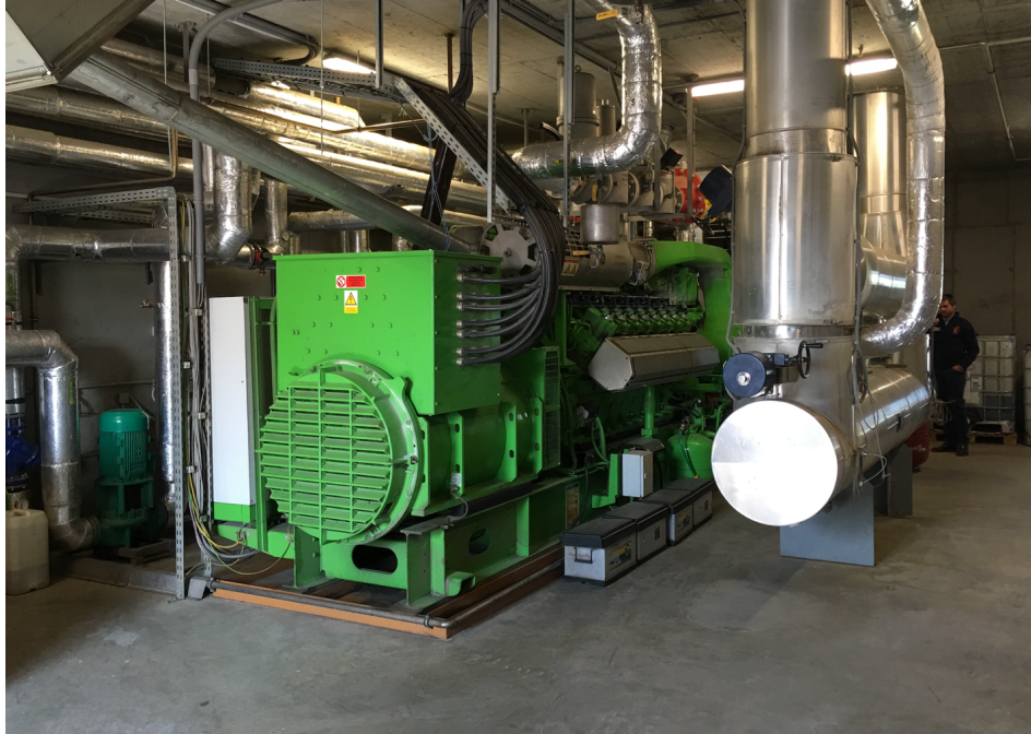
Figure 8 Biogas electricity generator in the Czech Republic
